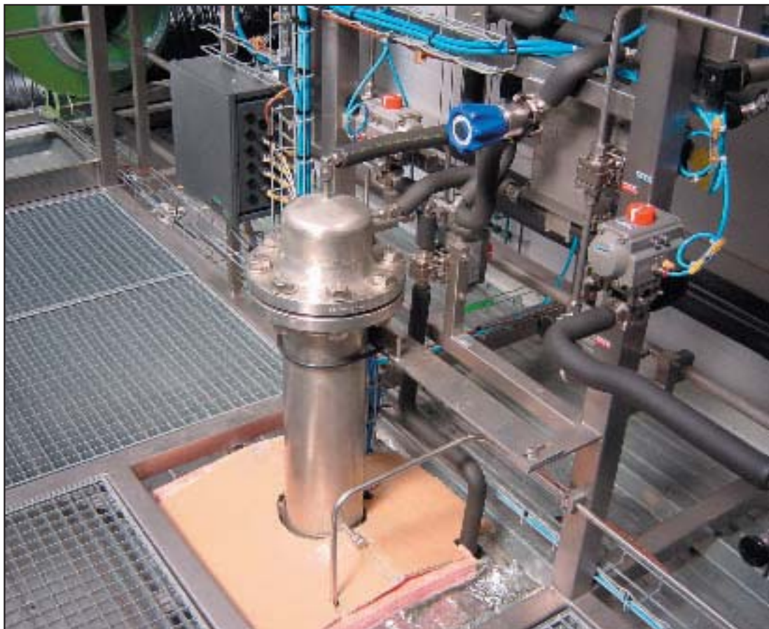
The distillation column passes through the roof of the process container.
